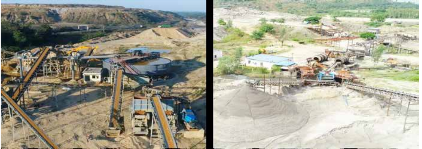
Processed Overburden Plant at Gonegaom Area by WCL & at Srirampur OC Mines by SCCL
