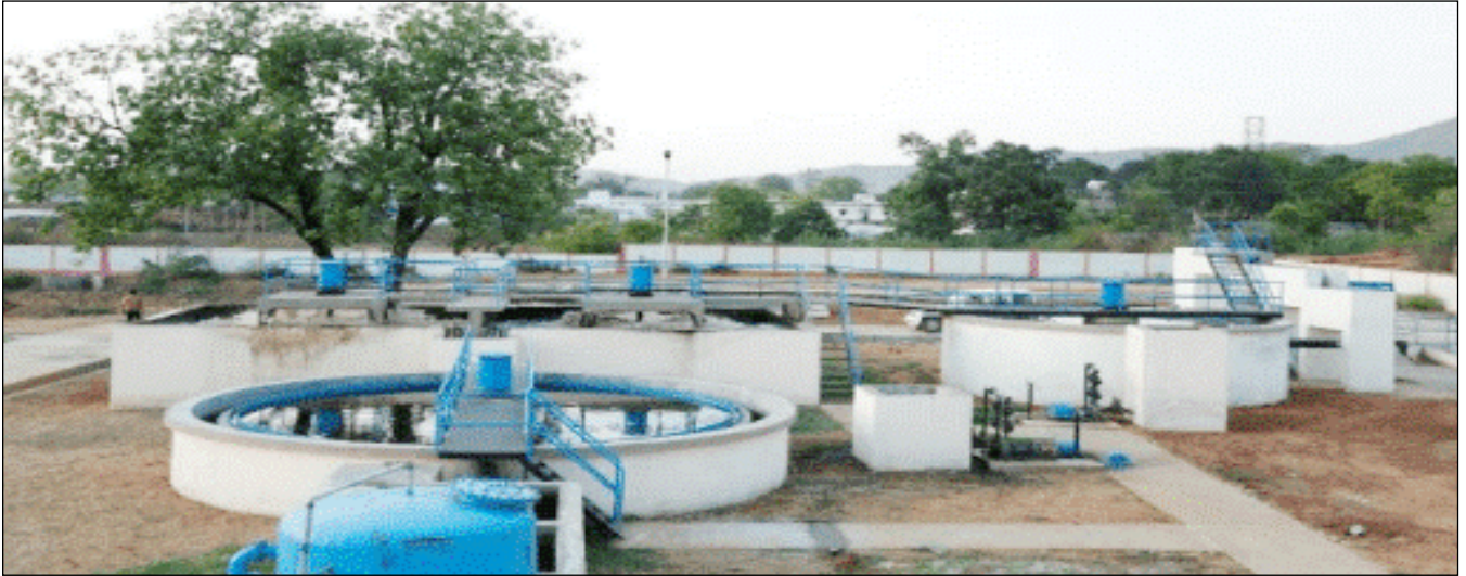
Fig. 0.8 MLD STP at Block-B, NCL
