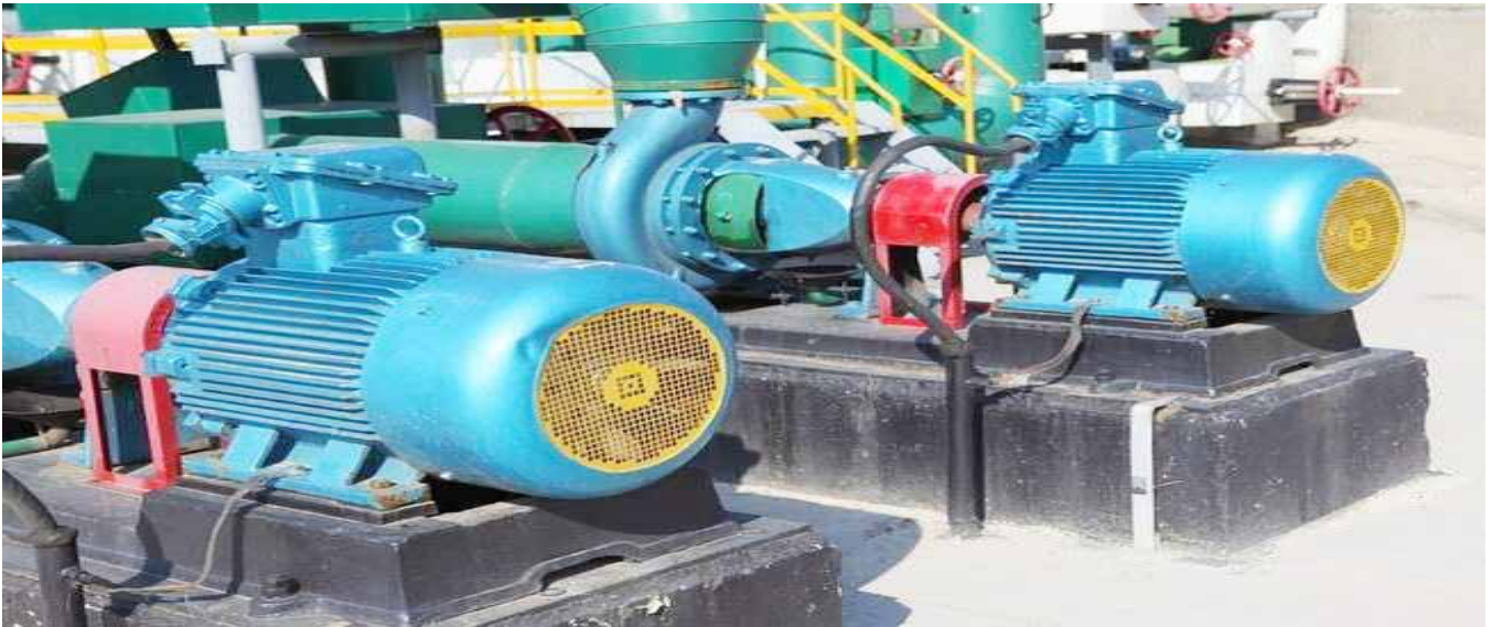
Pump House With IE3 Motor at SECL
