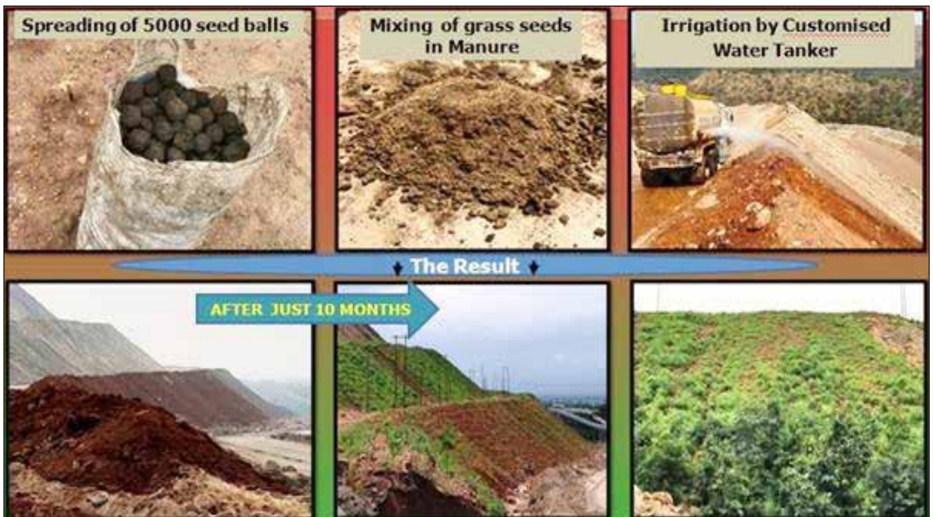
Steps taken for effective and sustainable plantation at Nigahi OC of NCL
