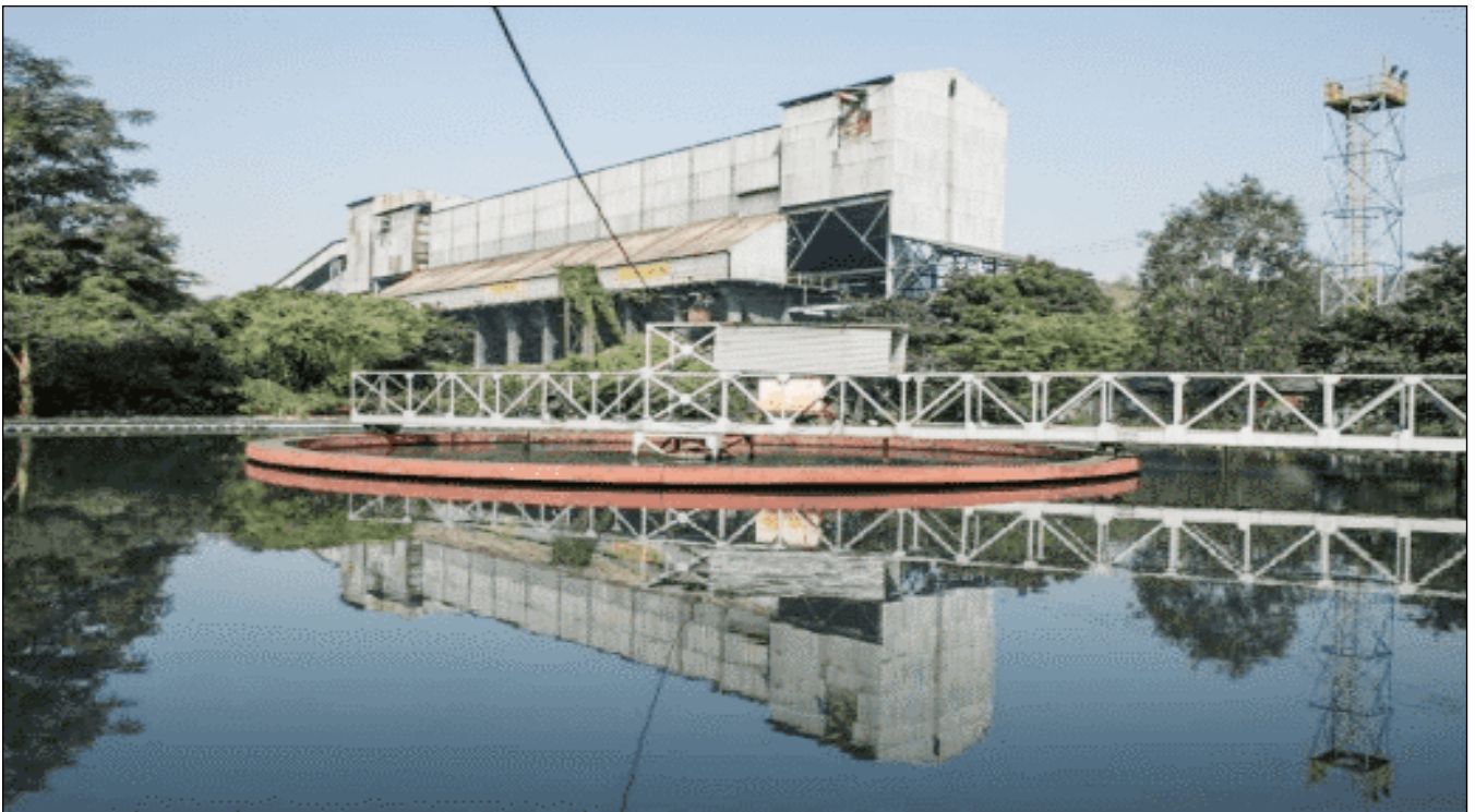
Fig. ETP at Kakri OCP, NCL
