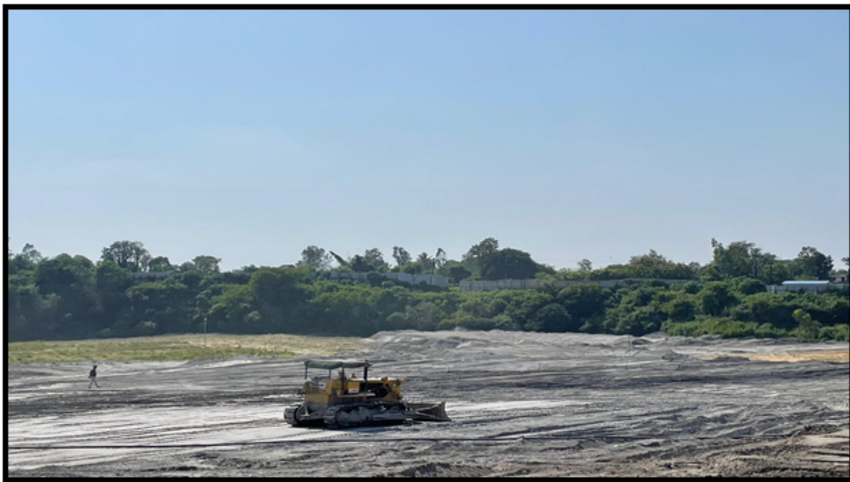
(Fly Ash filling at old Abandoned Quarry of Manikpur OC, Korba Area)
