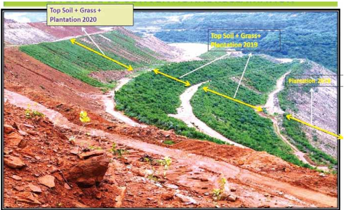
Fig. Steps taken for effective and sustainable plantation by grassing at Nigahi OCP, NCL
