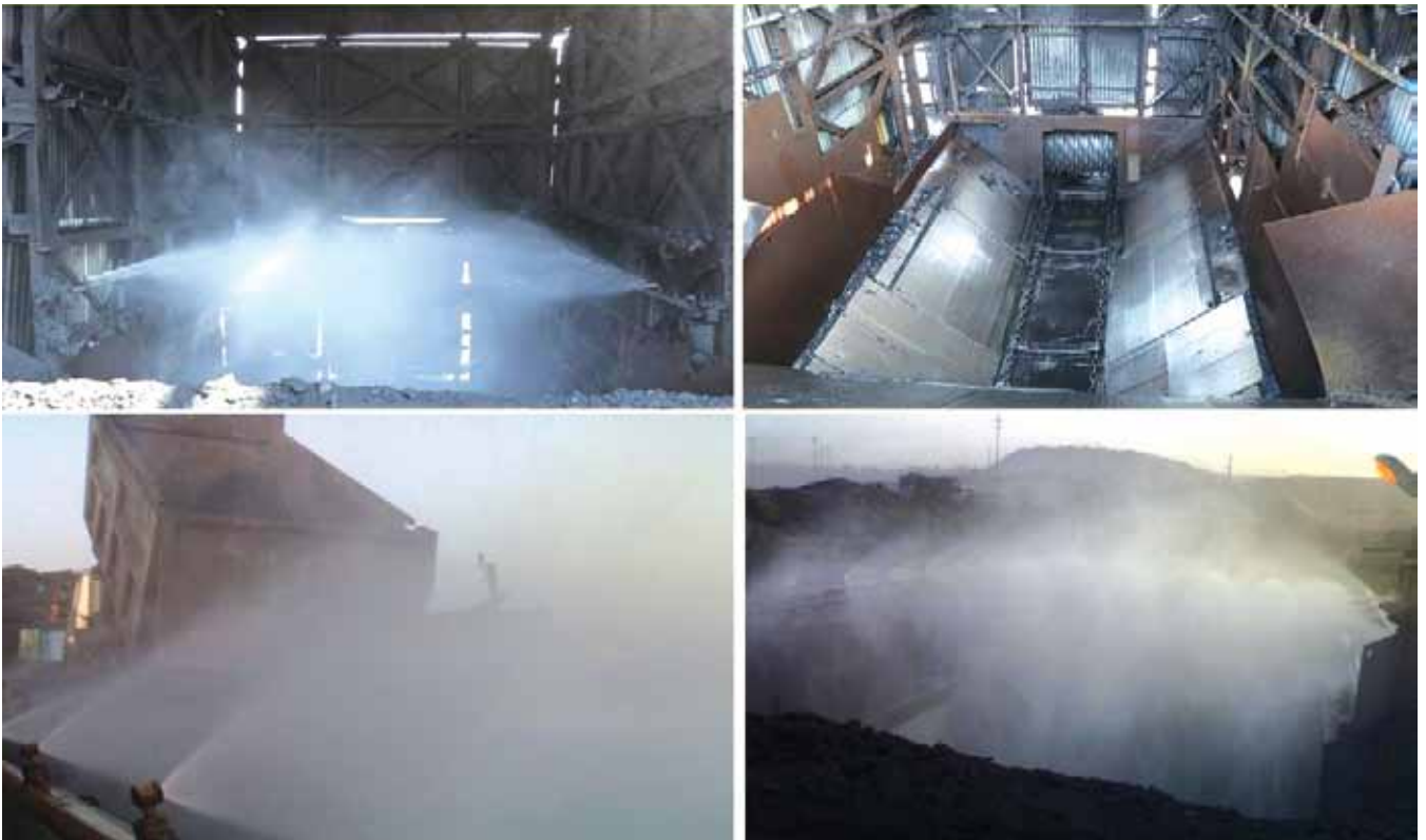
Fig. Feeder Breaker with Mist Spraying Arrangements at Gevra OCP, SECL
