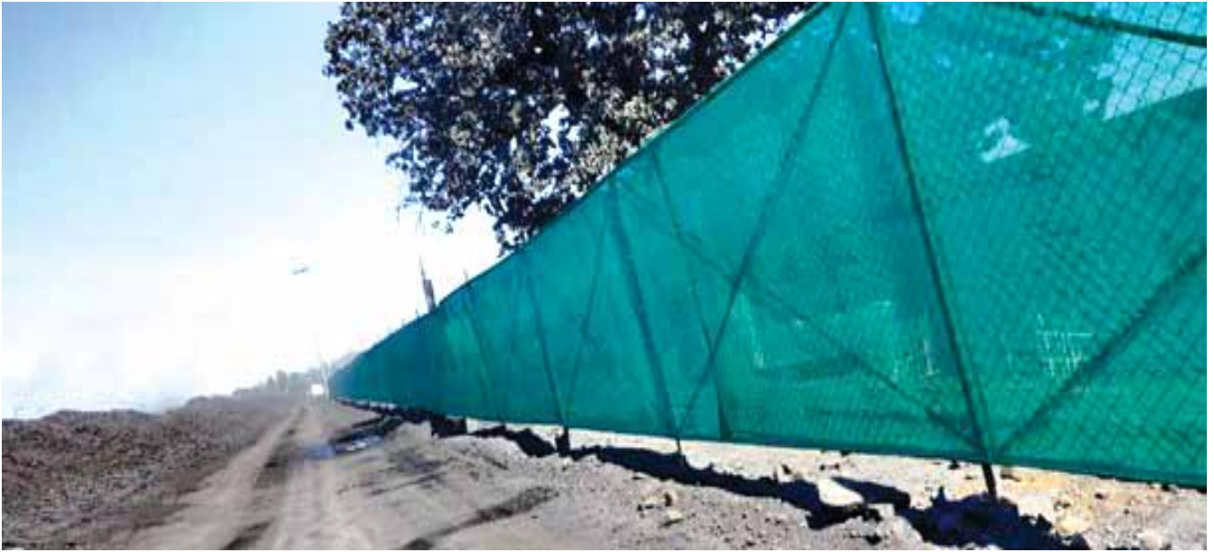
Fig. Wind screen at Phulbasia Siding, Magadh Area, CCL
