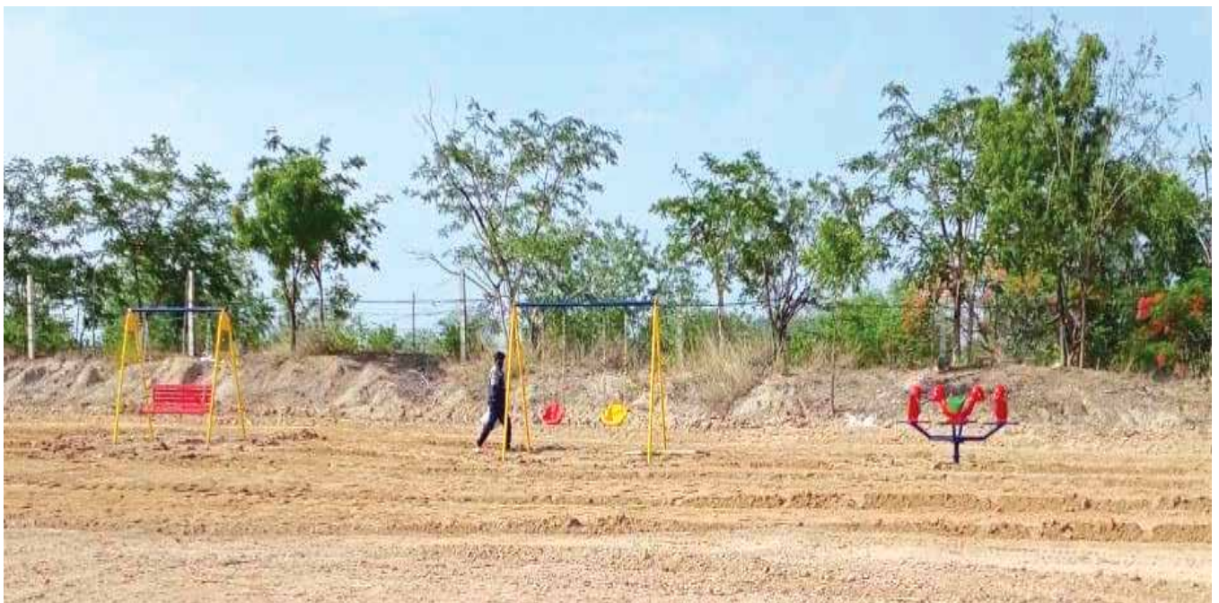
Fig. Children Play Equipment installed at Mine-II Eco park
