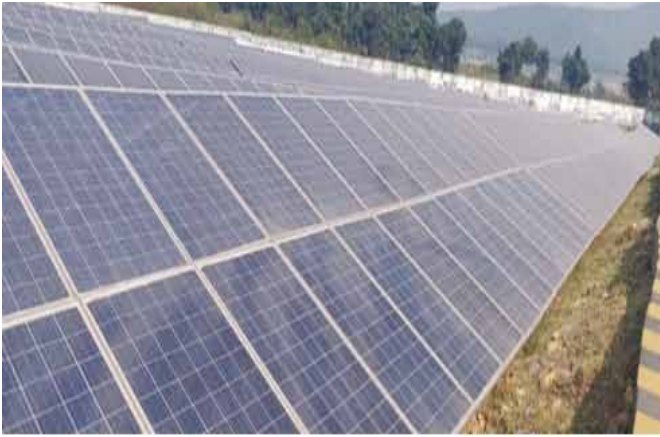
Ground mounted Solar plant in MCL
