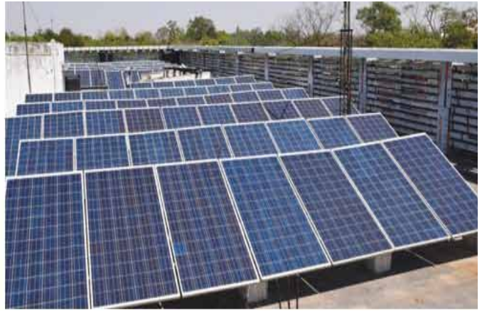
Roof top Solar plant in CCL
