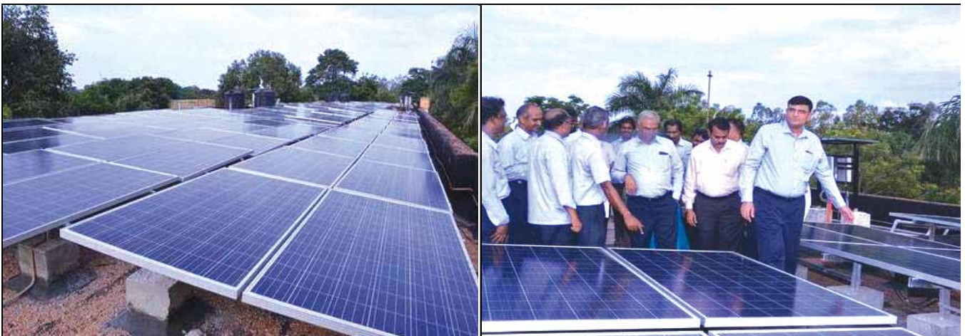
Fig. Roof Top Solar Power Panels on Residential Building at Neyveli, NLCIL
